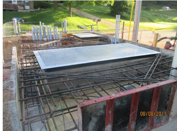
View of the top section of the Bowen Street lift station with hatches and electrical conduit in place.
